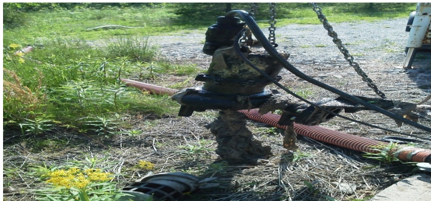
The pump shown from the Rolling Acres lift station was destroyed by the "flushable and disposable" wipes seen hanging from the impeller.
