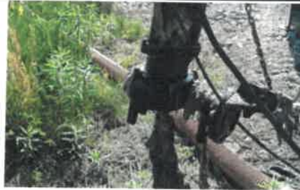
The pump shown from the Rolling Acres lift station was destroyed by the "flushable" wipes you can see hanging from the impeller.
